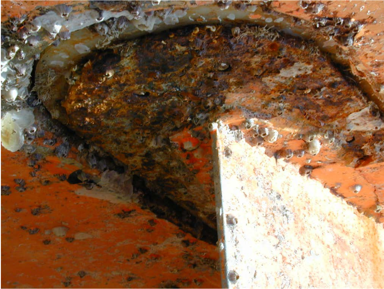
Galvanic corrosion at aft end of the keel spar Possible contributor to loss of the bulb?
